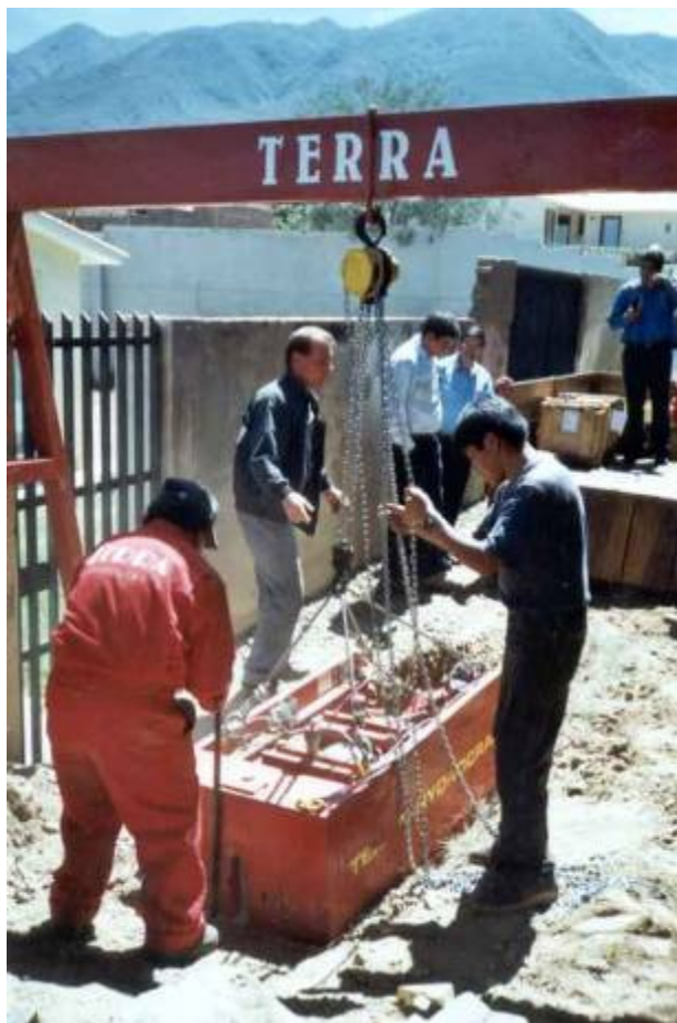
Picture above left: The TERRA-HYDROCRACK HC 600 S is lowered into the pit.
