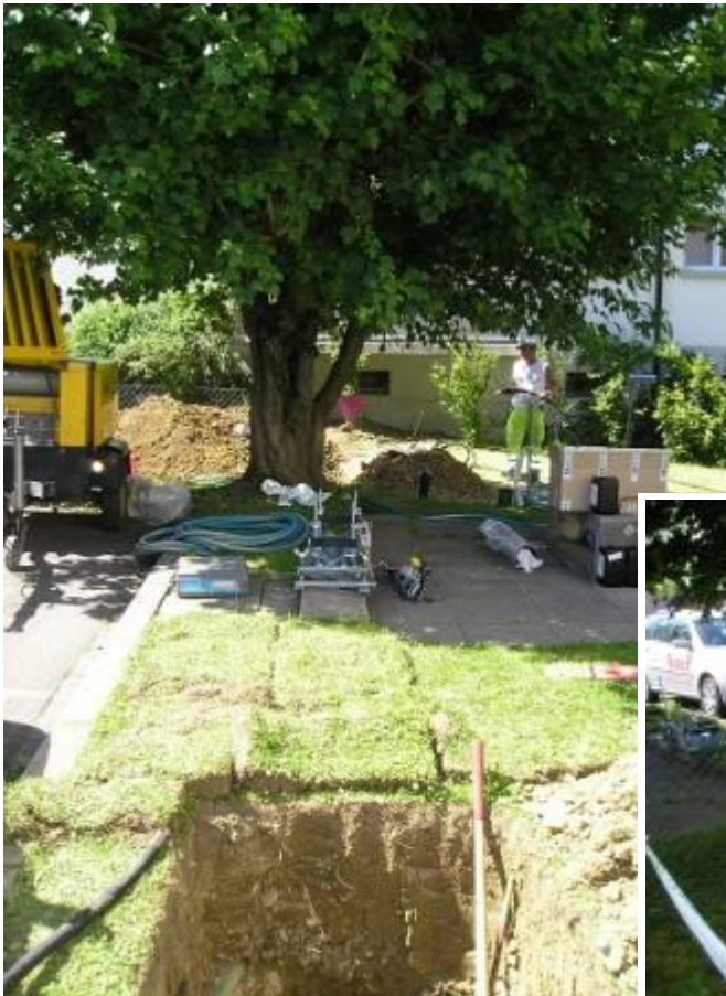
View onto a typical jobsite: limited space, old trees and green which should be damaged as less as possible.
