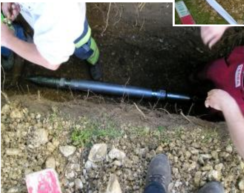
The TERRA-HAMMER TU 105 S/KOK-LD in the starting pit. Due to limited space the launching cradle could not be used. From this pit 2 parallel bores had to be done.
