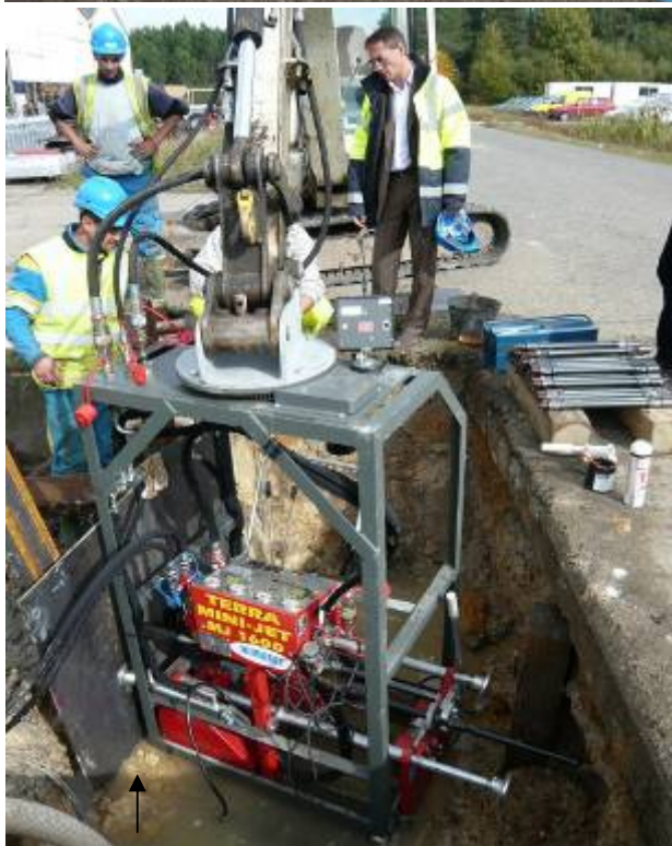
↑ The TERRA MINI-JET MJ 1600 with excavator frame during the back reaming and pipe pulling. The HDPE pipe OD 200 mm (8") is pulled in over a length of 47 m (155 ft)
