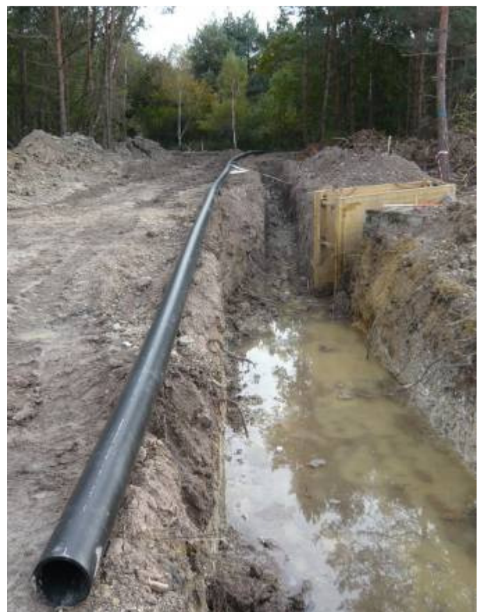
→ The 60 m (200 ft) long HDPE pipe OD 200 mm x 11.9 mm (8" x 0.5") is laid out at the arrival pit. It is ready for pipe pulling.
