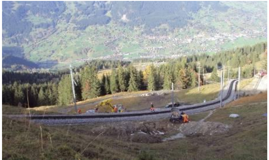
View onto the job site. The four pipes are laid underneath the rail way. In the background you can see the village Grindelwald.
