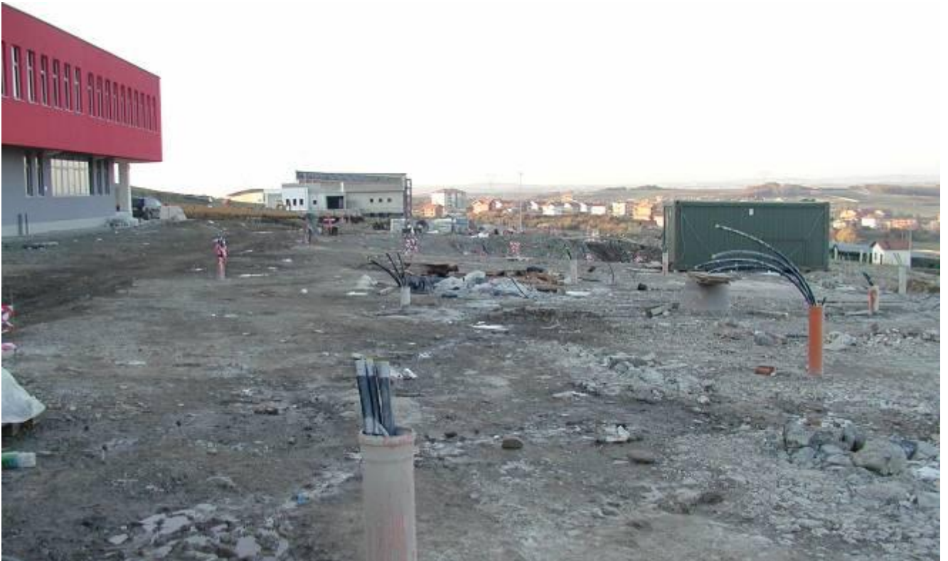
View at the first 15 successful bores. The first 15 heat sondes look out of the ground.
