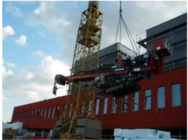
← The TERRA-JET 4407 V is unloaded with the crane. It weighs only 1.8 tonnes (4000 lbs). ↓
