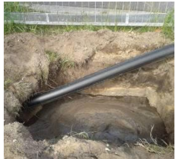
The HDPE pipe OD 125 mm (5") is pulled in. The drill mud with the sand flows into the target pit.
