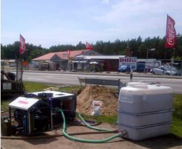
Power pack, mixing+pumping station and the 1'1000 ltr (290 gal) drilling fluid tank were placed besides the working pit.
