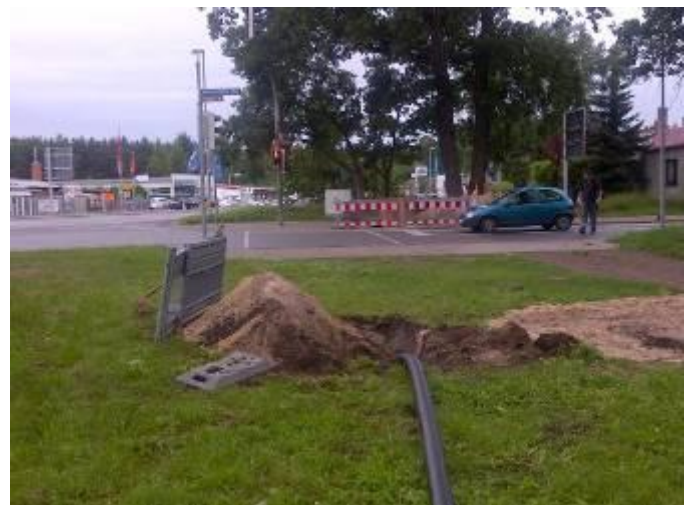
The HDPE pipe OD 125 mm (5") is pulled in underneath this road in a distance of 40 m (132 ft).
