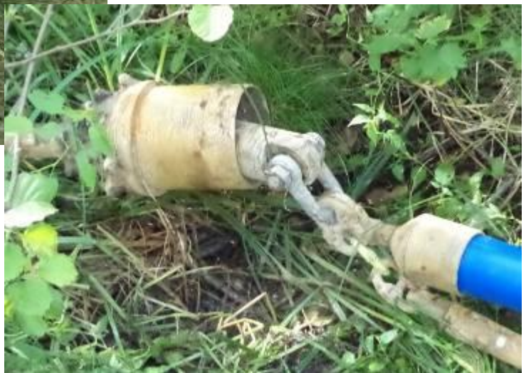
→ The backreamer \varnothing 260 mm (10") with the two HDPE pipes OD 110 mm (4.3") and OD 63 mm (2.5") just before backreaming.
