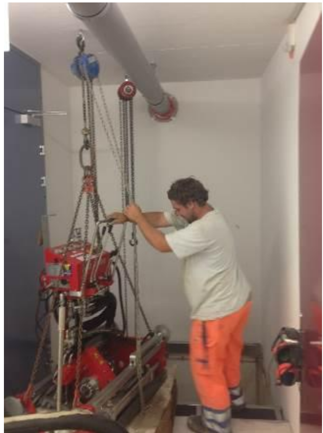
The drill rig is lifted into the drilling position with two chain hoists.
