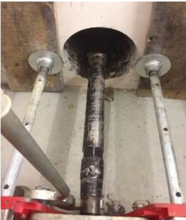
The drill rig TERRA MINI-JET MJ 1600 is installed. The sonde housing starts the bore.
