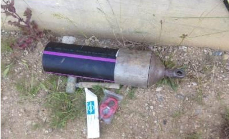
The first short pipe is pulled with an expander chuck. All other short pipes are screwed in the manhole.
