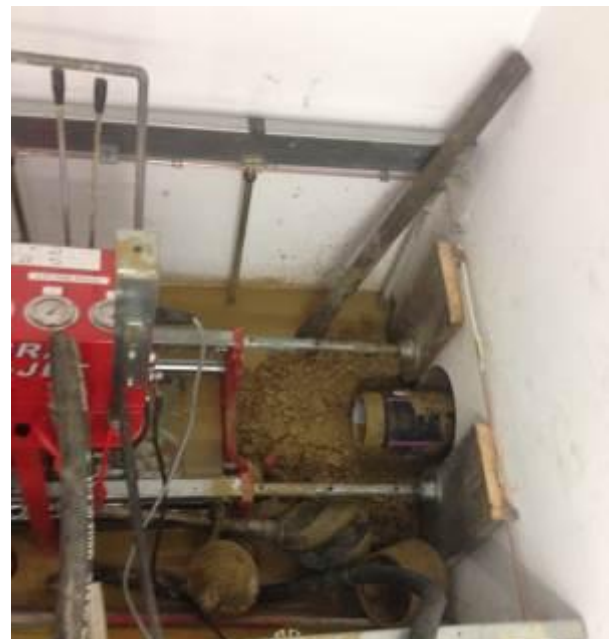
The new pipe has been pulled in completely. Then the core drill is filled with concrete.
