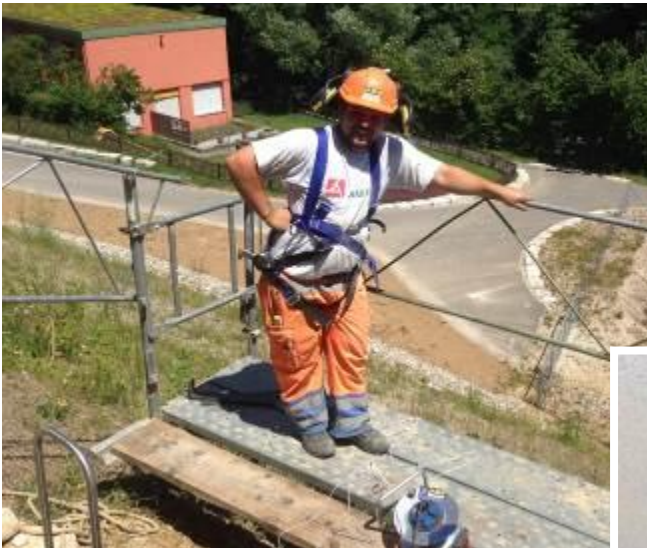
← The contractor Serge Jakob sets lots of value on safety. He is equipped with helmet, gas alarm unit and climbing harness.
