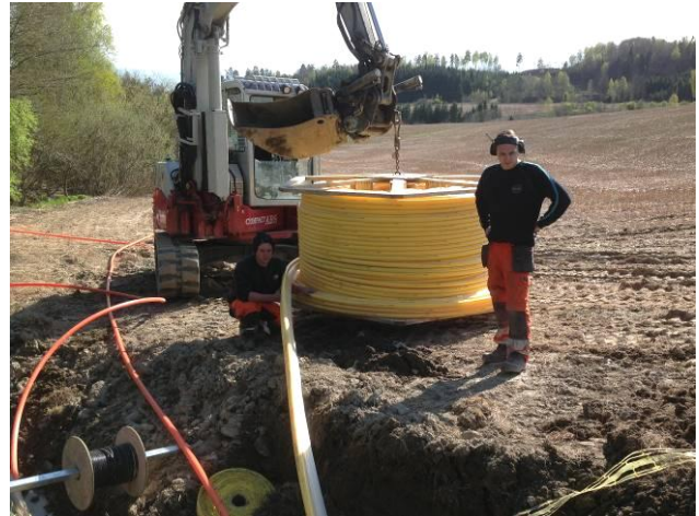
The pipes to pull in are prepared on a pipe decoiler hanging on the excavator in order to unroll smoothly during backreaming and pipe pulling in.
