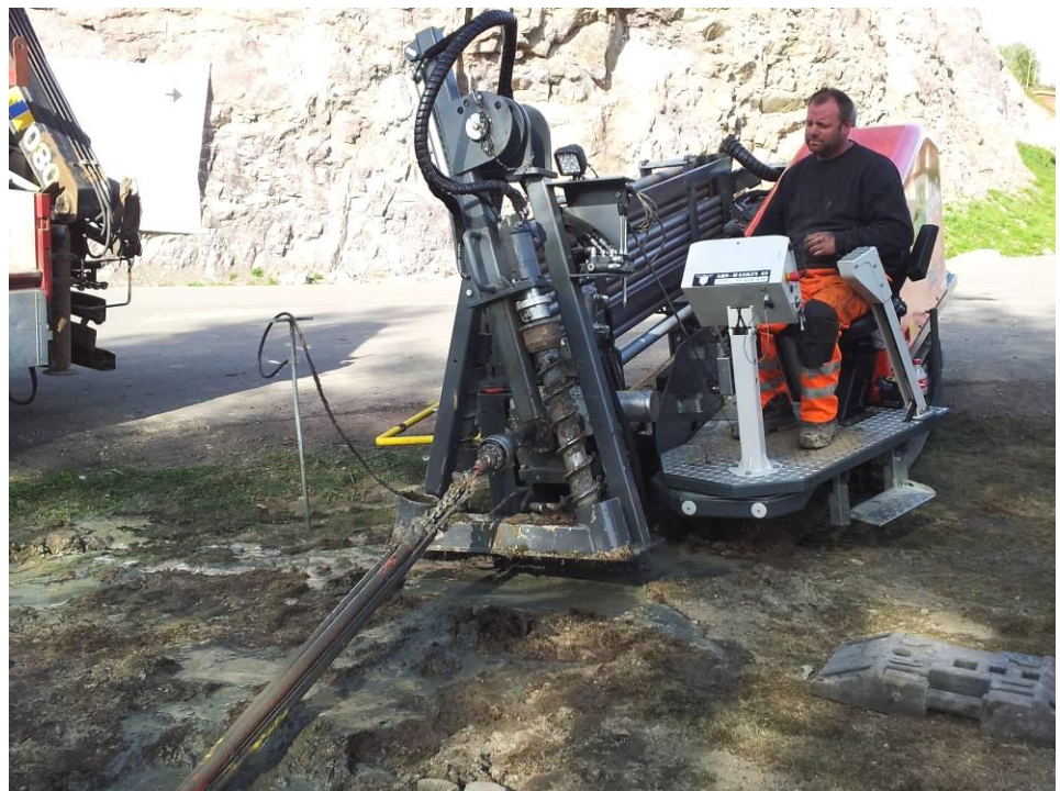
Owner and drillmaster Henrik Mikkelsen is pulling the pipes further back by driving backwards after a smooth and fast uninterrupted backreaming with simultaneous pipe pull-in.
