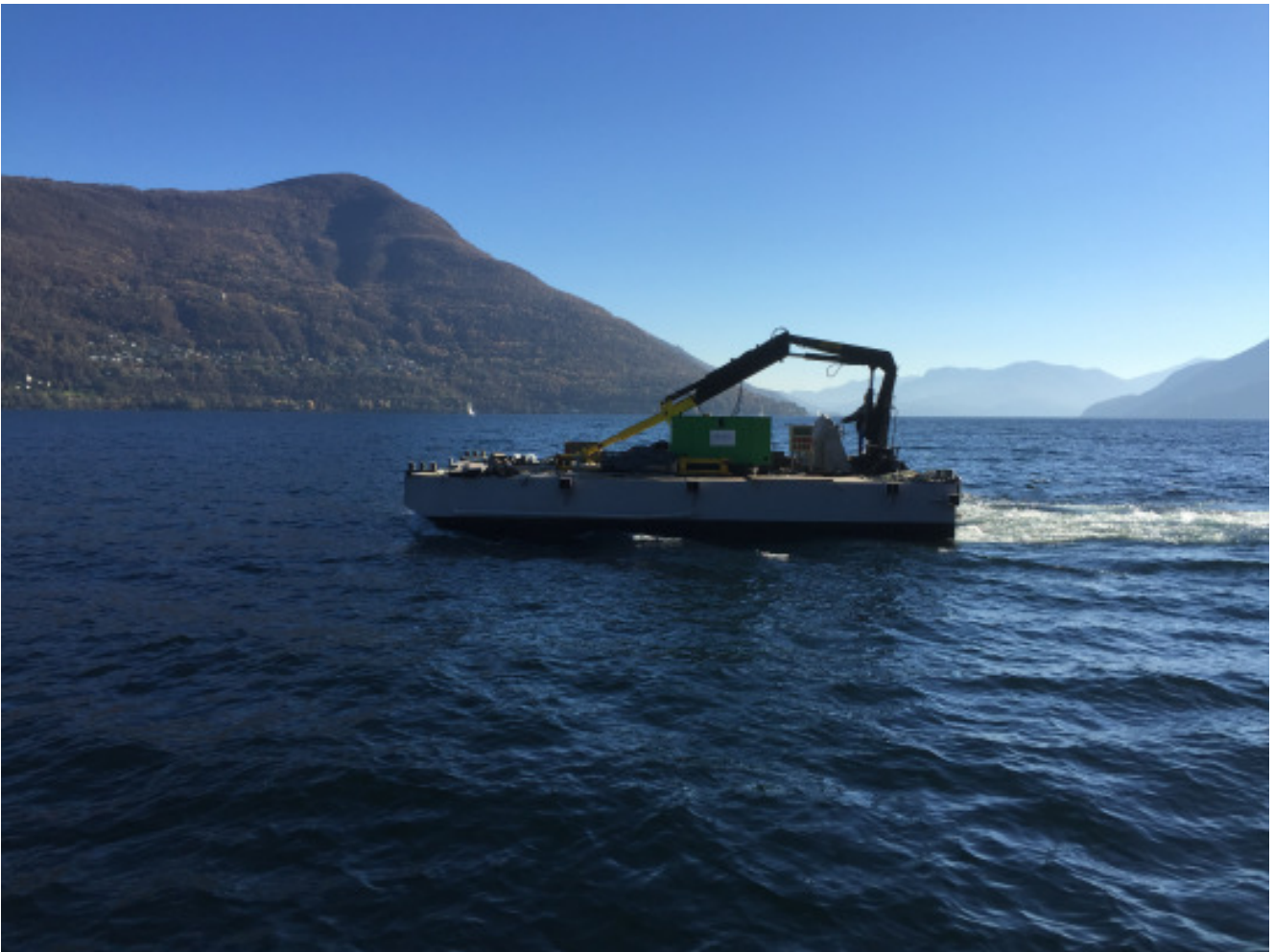
Pic. 1: The pontoon platform during the crossing of the Lago Maggiore. It is equipped with a crane, an air compressor and a generator. The new steel pipes and the ram had also been lifted onto the pontoon.
