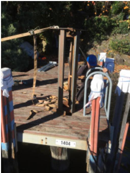
Pic. 4: For vertical alignment of the steel pipe a steel frame is screwed onto the old pier.
