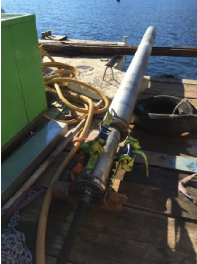
Pic. 2: The steel pipe, the ram ring and the ram were assembled and tightened with three tension belts. The pressure ring at the rear end of the ram has five lifting eyes.
