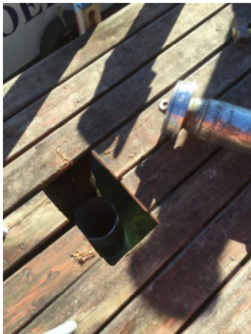
Pic. 6: The foundation pile is rammed in. Later on the new pier will be built onto this pile.
